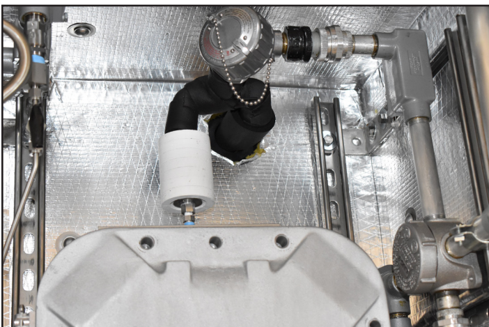
Figure 8 – Applying insulation to the VJT connections at the RTD and the Probe
