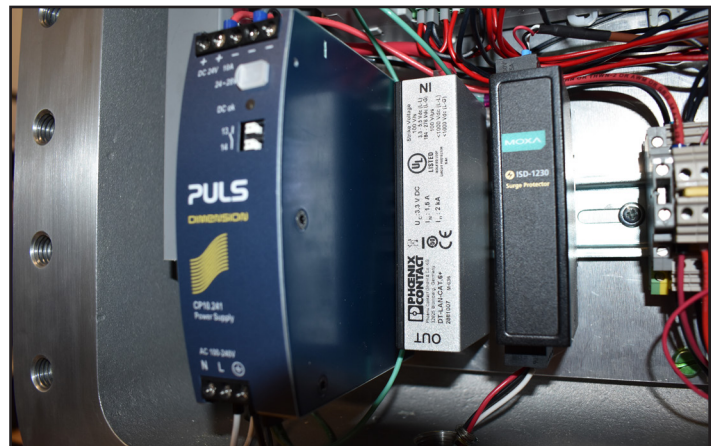
Figure 3 – Communications cable entry stub and connection point inside crock
